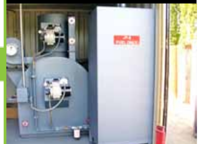
Therm-Tec Model CG-8 (Incinerator and Fuel Storage)
